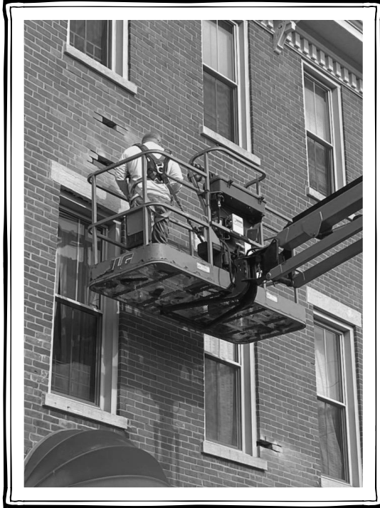
Rick Gass works on removing and replacing damaged bricks during the tuck-pointing project.
